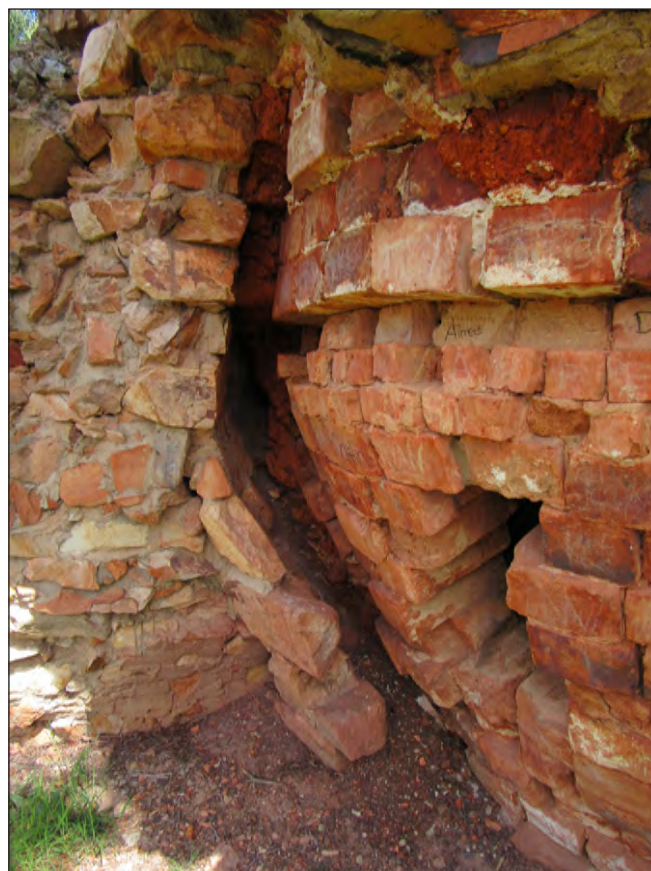
FIGURE 6: LAL LAL, THE SEPARATION OF THE FURNACE LINING FROM THE MAIN STRUCTURE
